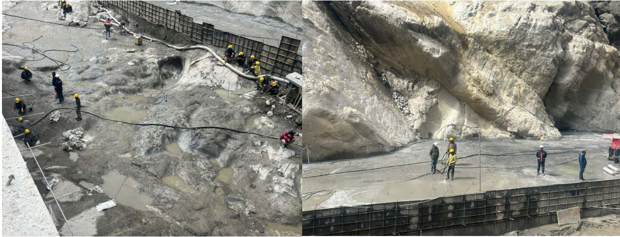
Manual cleaning of Rock surface in S3 block Green Cutting of concrete in S2 block with high pressure water jet
