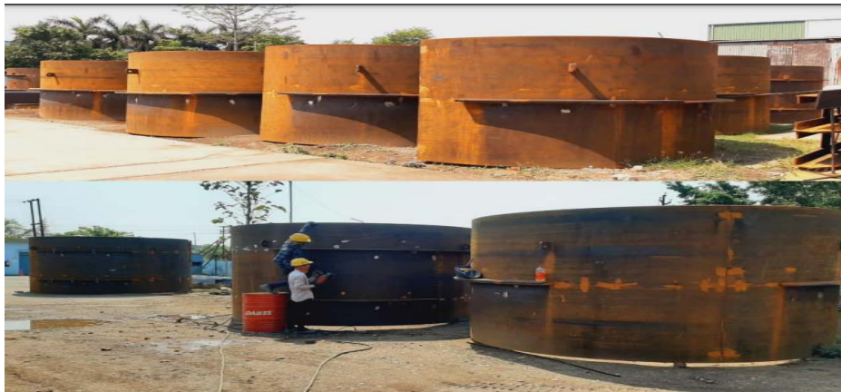
Fabrication of Pressure shaft liners has been started at Sitarganj (Uttarakhand) workshop of M/s PES Engineers Pvt. Ltd.
